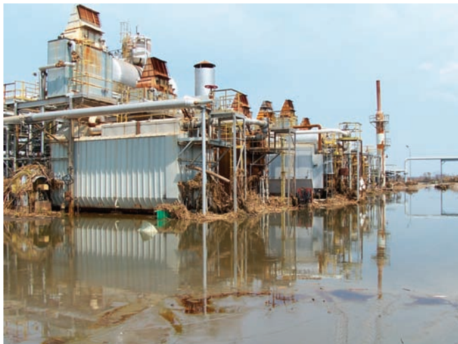
Natural gas processing plant in Louisiana flooded by Hurricane Katrina.
