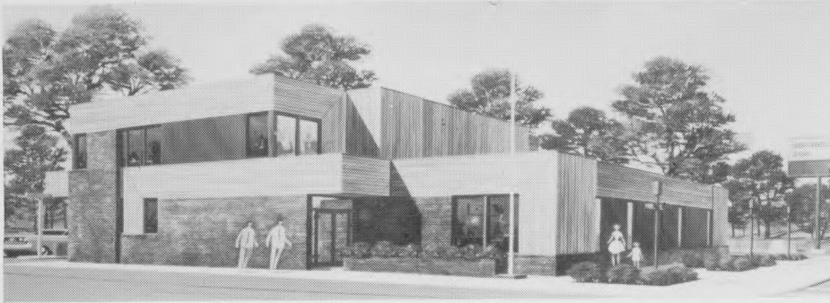
PICTURED above is a view of the northwest corner of the Northwestern State Bank of Dawson, now under construction. Besides the main level and second story mezzanine, there will be a one-third basement for storage and mechanical equipment.
