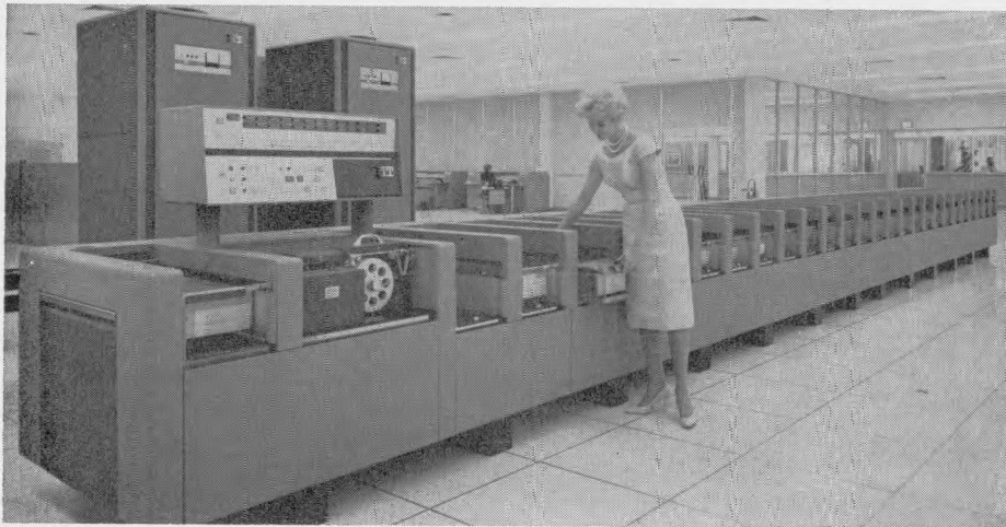
STREAMLINED FIGURE-R: Model Jo Ann Carley casts an approving eye at completely-automated electronic check handling and bookkeeping system installed by Valley Natl., Phoenix.
