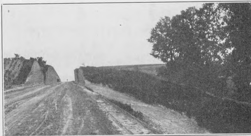
Soldier Road, Monona County, Iowa. The advantages of hill cutting are plainly evident in this picture. Since pioneer days, all traffic has climbed the one hill, coasted down the other side, then climbed the second hill, only to again coast down the side of the other. The modern road builder came along, cut his way through, took the dirt he cut away and piled it in the low flat beyond, raising the grade there to an easy grade with that he made through the hill. Now, for all time to come, traffic will haul its load of freight or passengers on an easy grade with no hill climbs. The height of the hill is indicated by the car and men in the cut. It looks like it might have paid to cut a tunnel through the hill, if necessary, to get away from the two heavy climbs to the top of the crests of these ridges which have barred the way.
