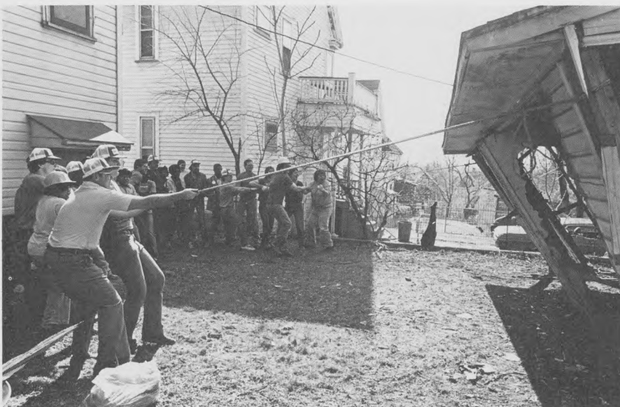
Bankers and local residents combine their efforts to pull down condemned garage during cleanup party at first house targeted for rehabilitation by Buckeye-Woodland Community Development Corp. Part of house is visible at left.
