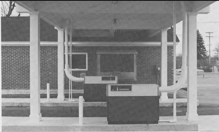
When water was discovered three feet below ground level, overhead LeFebure Tel-Air 1000 pneumatic-tube system replaced underground Tel-Air system originally destined for this facility of Northeast Bank, Sanford, Me.
