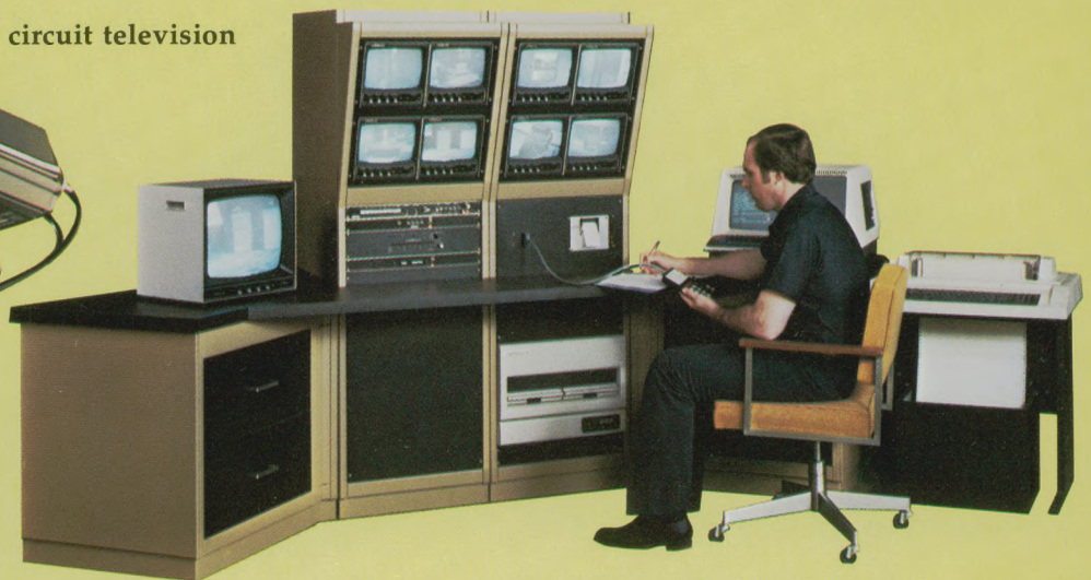
Central station/proprietary alarm system
