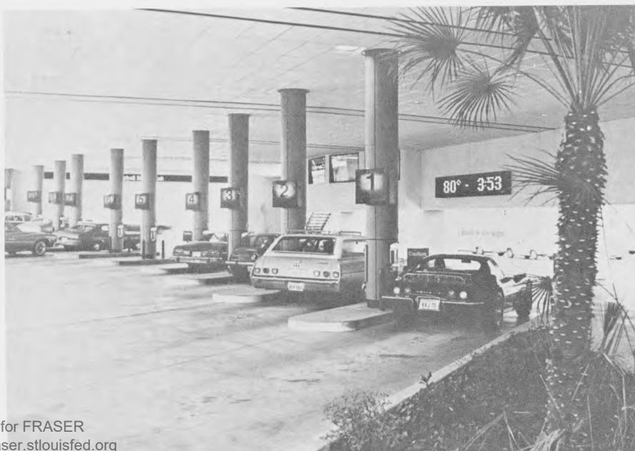
Drive-up installation at First City Nat'l, El Paso, Tex., features Mosler Pneu-Vista® 3 System, which allowed bank to save thousands of dollars in trenching costs. This up-send system sends carriers to overhead teller station, under which drivers pass after completing transactions.
