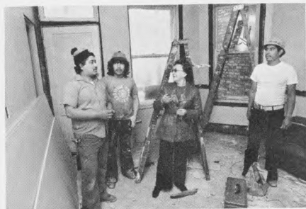
Typical NHS rehabilitation project carried out by rehabilitation and financial counseling from Neighborhood Housing Services. Establishment of new NHS office in Chicago's Little Village neighborhood will be financed by $375,000 pledge from Continental Bank Foundation.
