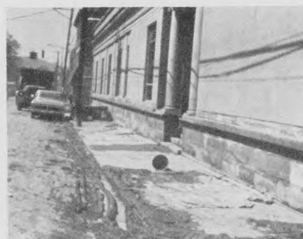
This is exterior of bank building after flood was over.
