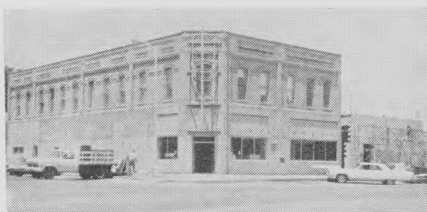
As Phase 1 (r.) of First of Perry's construction was being carried out, second phase was prepared for by removing facade from original bank building (l.) before demolition.
