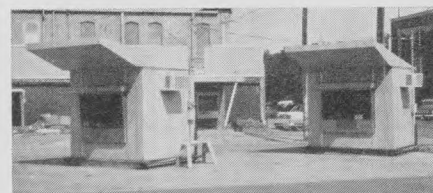
Temporary drive-up units (foreground) were used by First of Perry during construction of new quarters. In background, old drive-up units are dismantled. New building's drive-up facilities feature LeFebure model 2111-T electric drive-up window and Tel-Air 9 remote pneumatic kiosk units. Additional LeFebure equipment includes under-counter equipment, walk-up window, night depository and complete alarm components.
