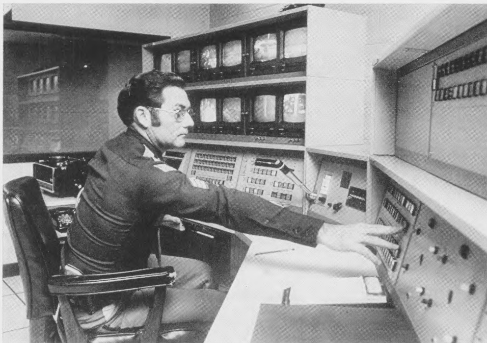
Sgt. Charles Hale of Fort Worth National's guard force sits at console of bank's central surveillance and control console. TV monitors show what is going on in all areas of bank. Access to critical areas is controlled by magnetic door switches.
