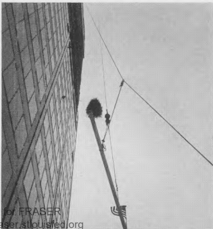
Almost there! Beam with cedar tree and American flag nears top of new First National tower.
