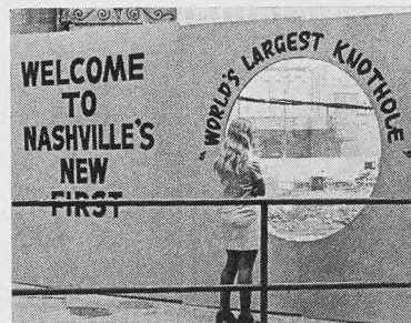
Pretty sidewalk superintendent takes advantage of the "world's largest knot-hole" in the barricade surrounding the construction site of First American National's 28-story office tower and interlocking four-story banking center. The project is being developed by First American National and Equitable Life Assurance Society of the United States.
