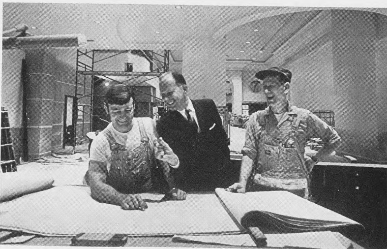
The ABA vice president visits American National's upper banking floor, which is being completely remodeled in warm, classic Williamsburg decor. Mr. Stults keeps a daily eye on each detail of the remodeling and reconstruction.
