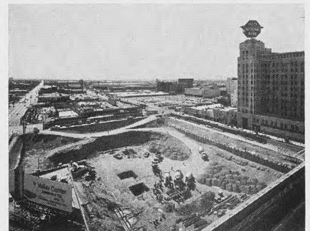
The first cement footings are poured for the new Valley Center in Phoenix. When completed in the fall of 1972, the financial headquarters for Valley National will rise 40 stories.
