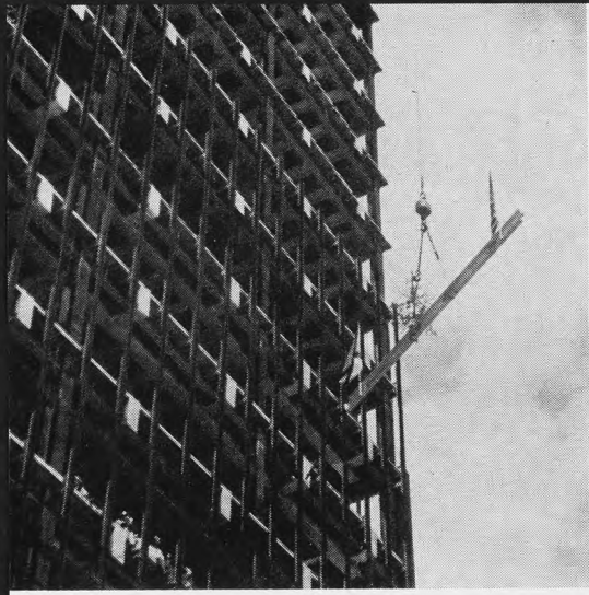
TOPPING OUT at First of Birmingham saw this 28-foot beam (and tree) hoisted into place.
