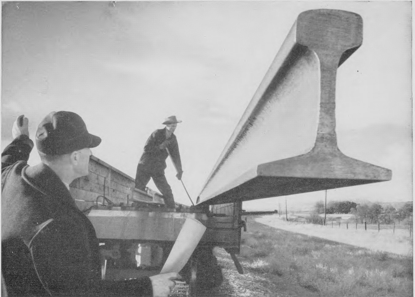
JUTTING ABRUPTLY from the rear of a Northern Pacific work train near Big Timber, Montana, this 38-ton length of rail is about to be lowered into place on the ties. As a crane holds the rail, the train pulls out from under its load.
