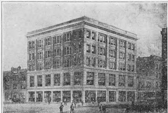
New home Northwestern Trust company and Scandinavian-American bank of Grand Forks, N. D., now under construction.
