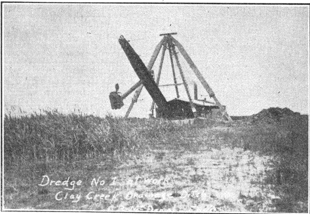
Digging the Big Clay Creek Ditch in Clay and Yankton Counties, South Dakota.
