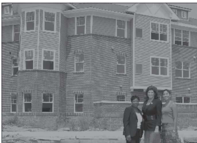
From left, Ruby Bright, executive director of the Women's Foundation; Susan Stephenson, board chair of the Women's Foundation; and Karla Davis, project manager of Memphis Hope in front of the construction site for Phase I of University Place, which is almost complete.
