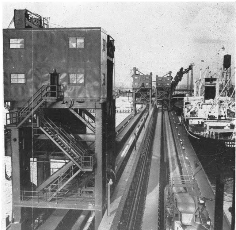
—Through the courtesy of the League of Virginia Counties Pier 14 at Newport News. The new low-level C. & O. pier is equipped with multiple belt conveyors.
