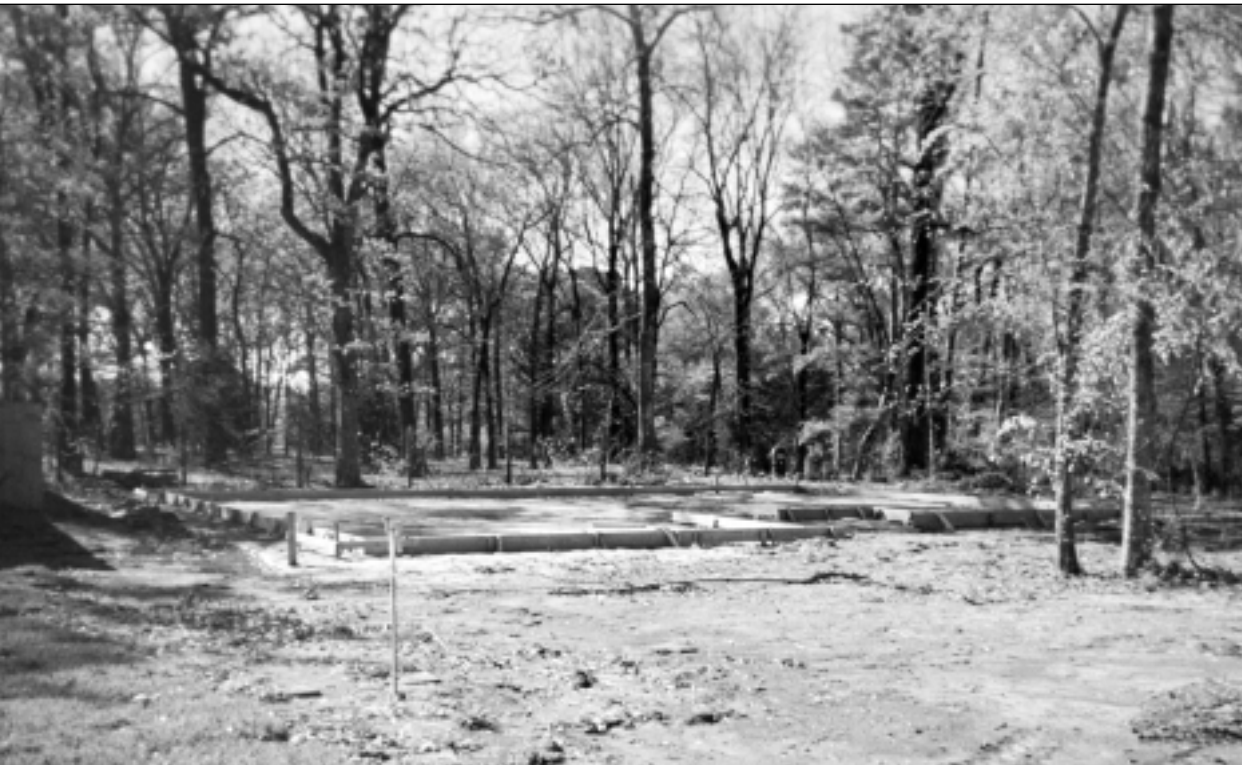
A foundation is ready to be poured for a house in the Green Oaks subdivision. Steve and Roxan Harris, who own H&H Builders, bought these 18 acres of woods in Nash to build an affordable housing subdivision.
