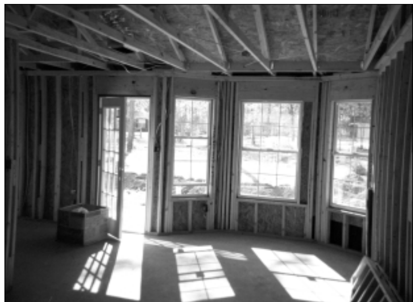
A public/private partnership came together to construct 69 affordable homes in the city of Nash.
