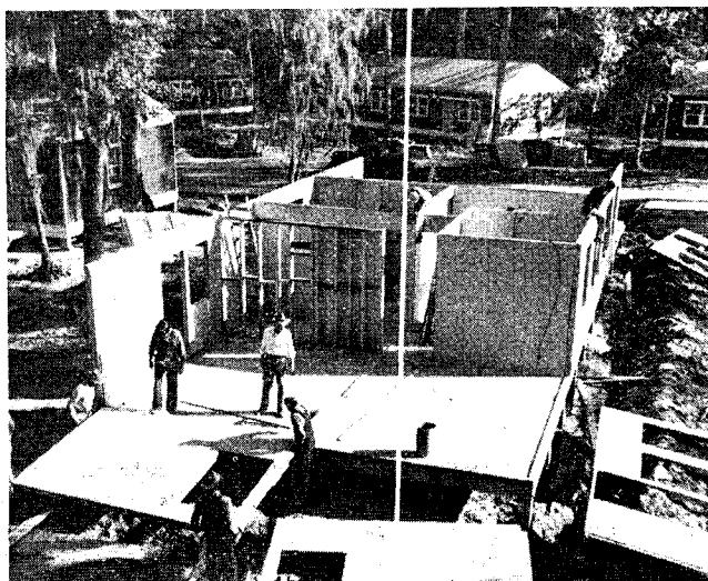
Six rooms, six hours, ten men. This factory prefabricated house in Liberty Hills, Charleston, South Carolina, was erected between 9 a. m. and 3:20 p. m.
