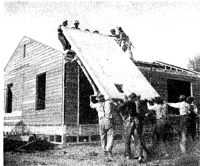
This photograph shows site fabrication at Barlow Place in Portsmouth, Virginia. The hole in the roof section is for the chimney flue.
