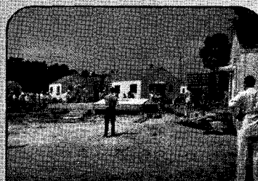
10:30 a. m. . . . Last pieces to be placed on truck were the floor sections and steps.
