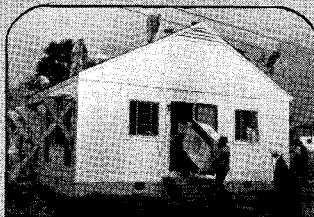
8:00 a. m. . . . While roof is loosened in sections, household equipment is being brought out.
