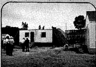
9:20 a. m. . . . All down, roof sections are ready to be loaded into a waiting truck.
