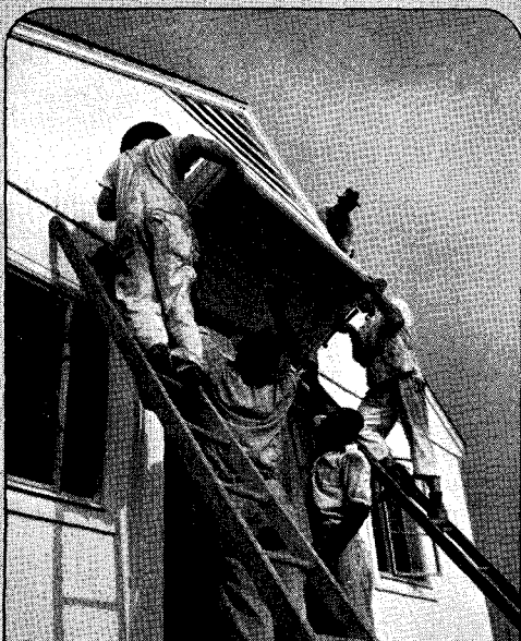
7:48 a. m. . . . Exterior decorations come off first. Workmen are here removing partition.
