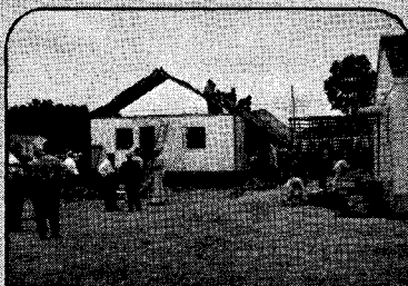
8:45 a. m. . . . Roof sections are easily handled by six workmen, who guide it down.
