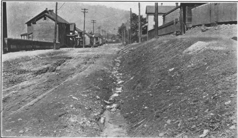
AN OPEN DITCH ALONG NEW STREET, PROSPECT.
