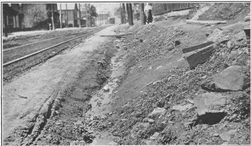
OPEN DITCH ALONG WOODVALE AVENUE, WHICH RECEIVES ALL KINDS OF HOUSE DRAINAGE.
