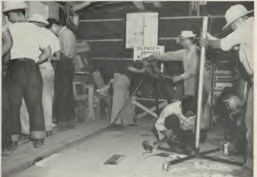
FIGURE 130: Diversified outlets for mechanical skills provided work with pay for many evacuees in the Assembly Centers. A group of mechanics welding an upright in the plumbing shop at Fresno (California) Assembly Center.
