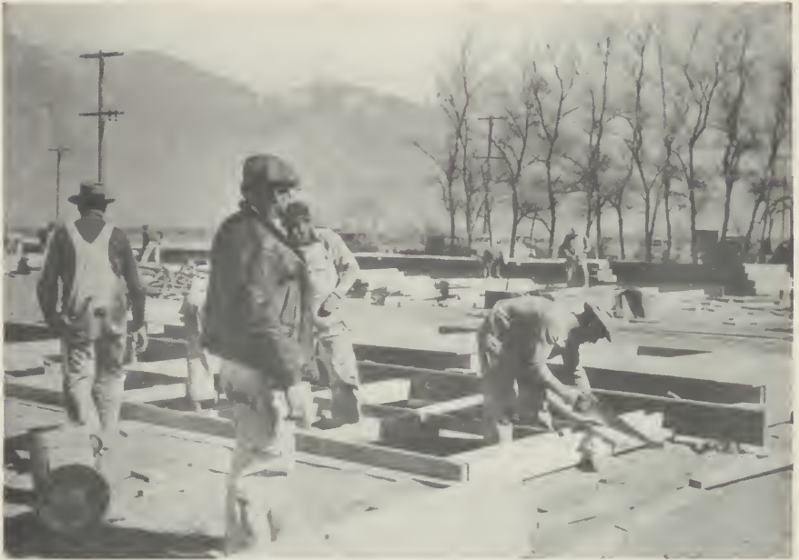
FIGURE 1: An early construction scene at Manzanar Reception Center, in Owens Valley, Inyo County, California. This was the first of a series of Centers constructed by the Army, and later became a Relocation Center under the War Relocation Authority.
