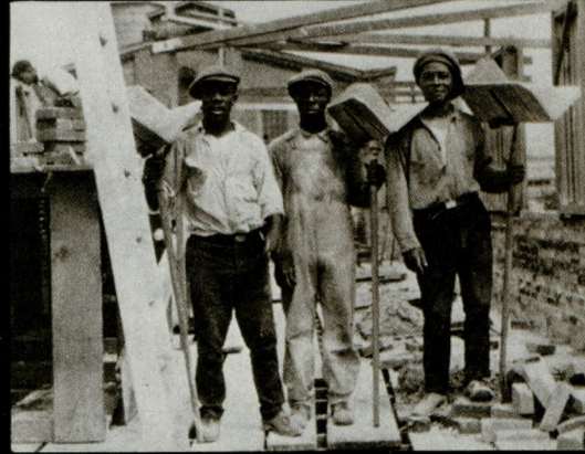
Hod carriers (brick-layers' assistants) at work. (Photo courtesy Temple University Libraries, Urban Archives Center)
