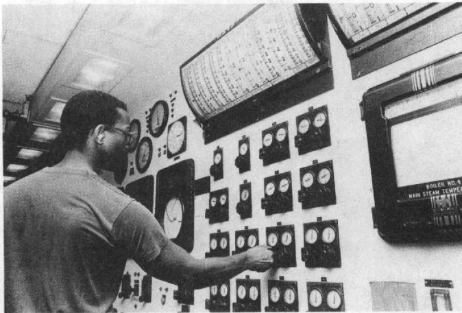
Power dispatchers make adjustments to generator control settings.
