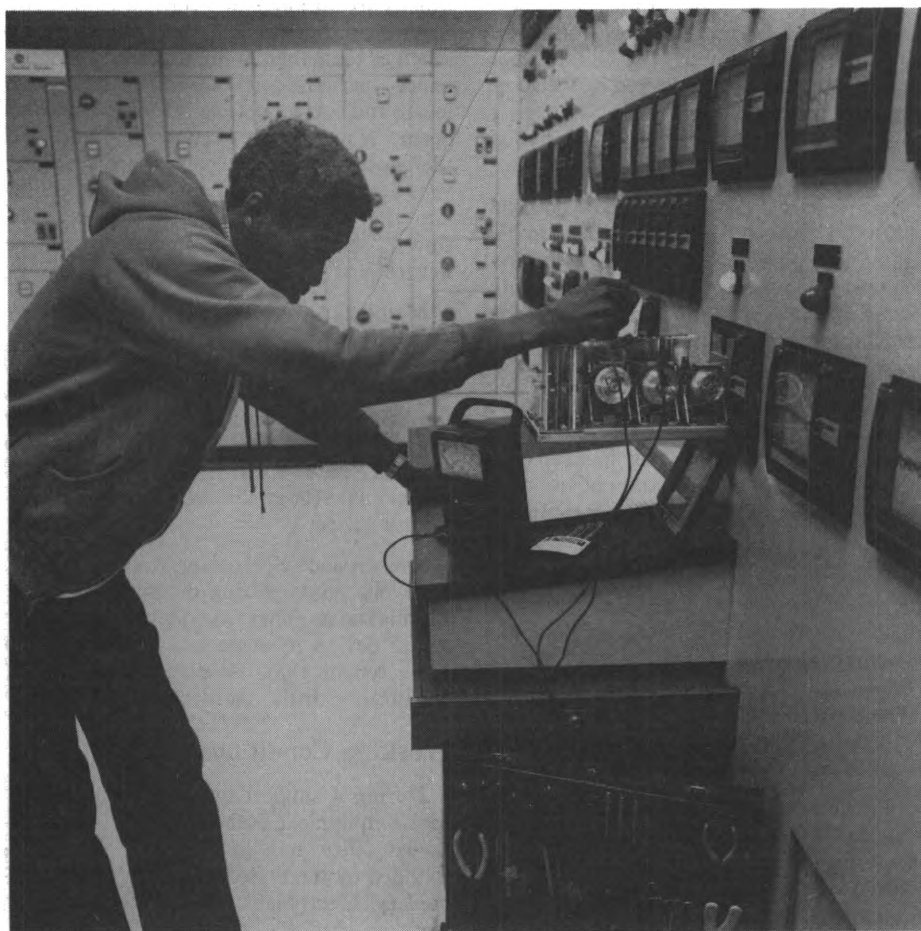
Maintenance electricians frequently use instruments to check equipment.
