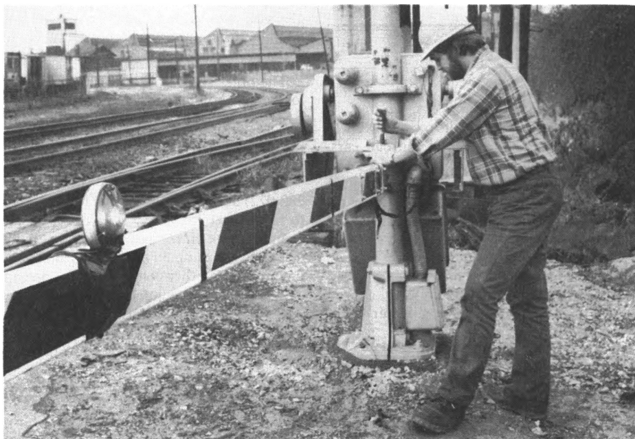
Signal maintainer inspects grade crossing.
