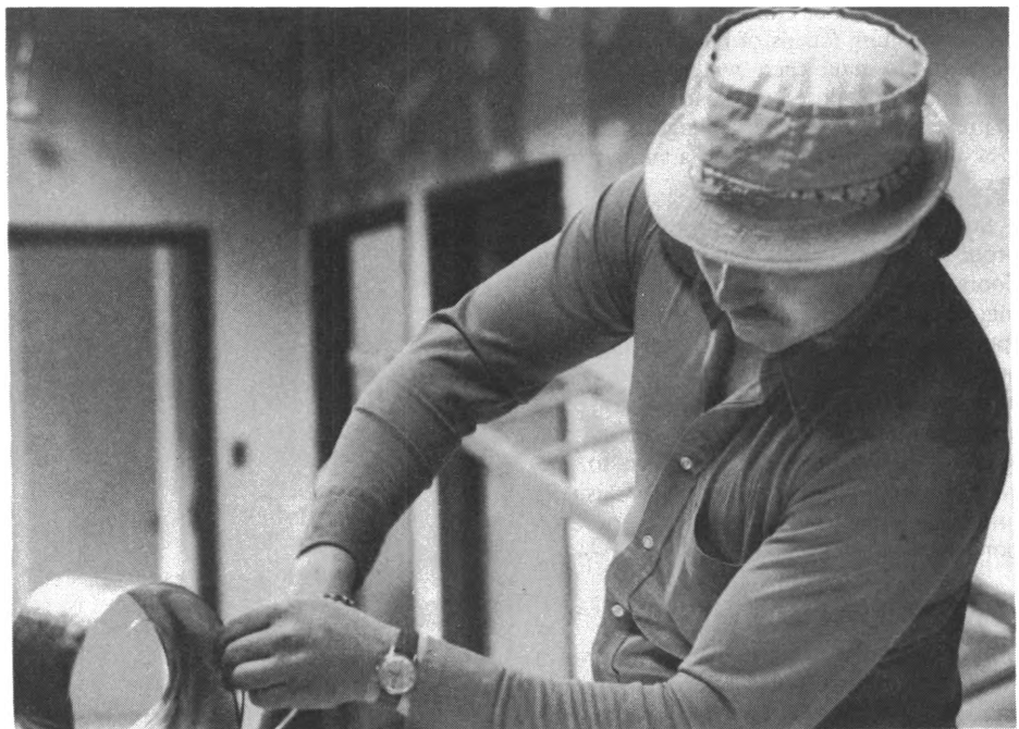
To insure proper fit, sheet-metal workers make corrections at the job site.
