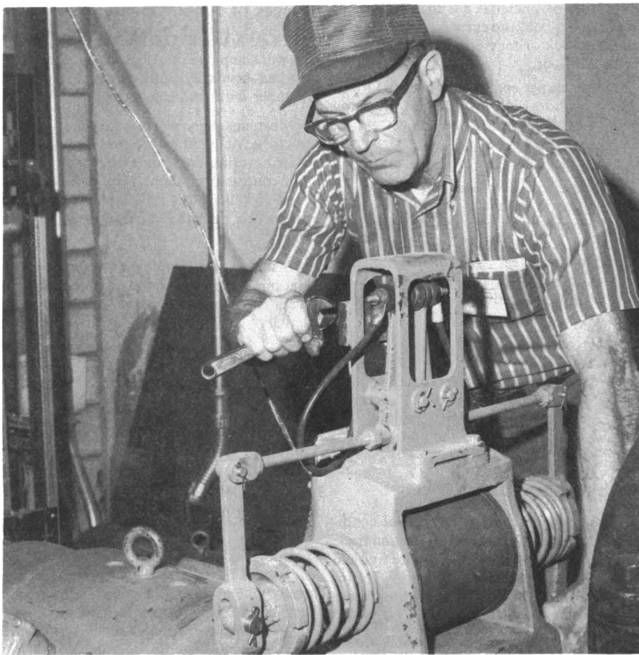
Elevator constructor retightening winch bolts loosened by vibration.
