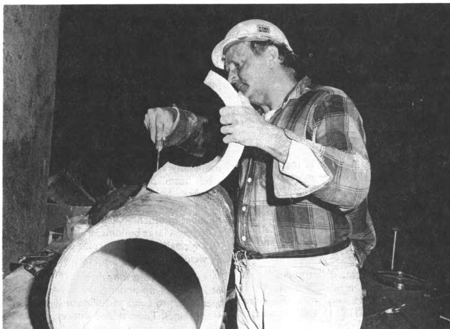
Insulation must be trimmed so it will fit over a pipe connection.
