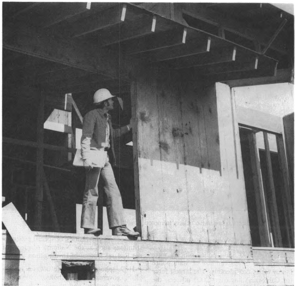
An inspector making sure the methods and materials used in the construction of this house meet the local building code.
