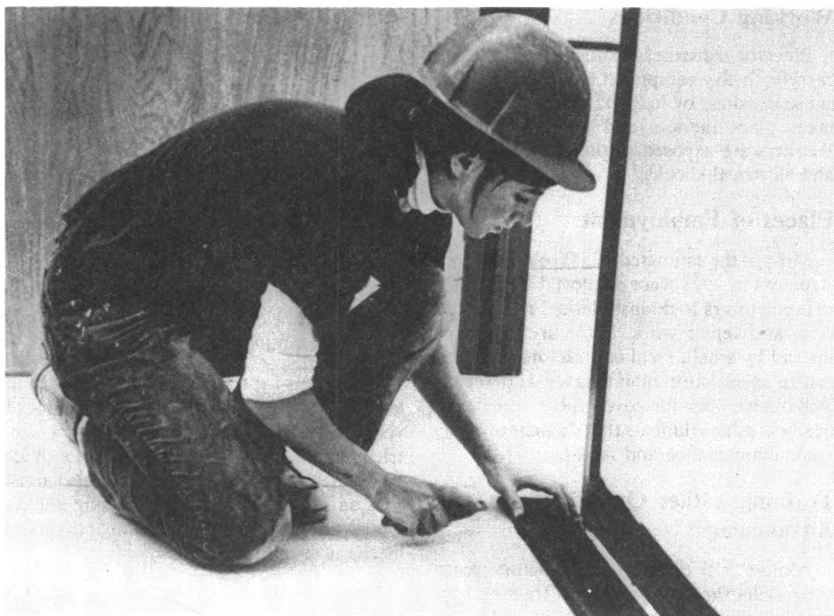
To complete a job, this floor covering mechanic measures, cuts, and glues vinyl molding along the bottom of the wall.
