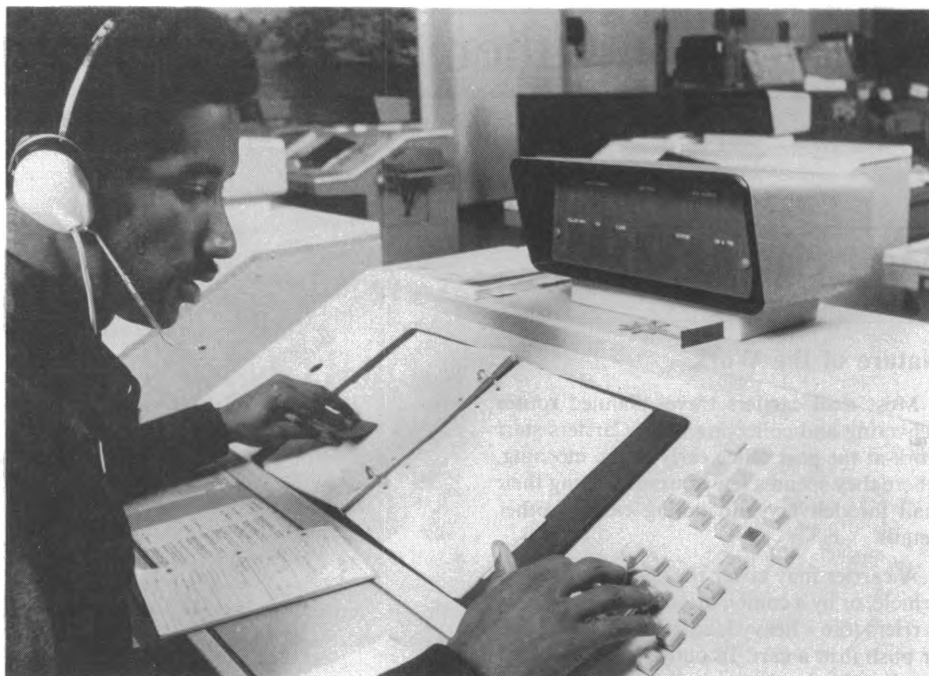
In many telephone company central offices, manual switchboards have been replaced with sophisticated computerized equipment.
