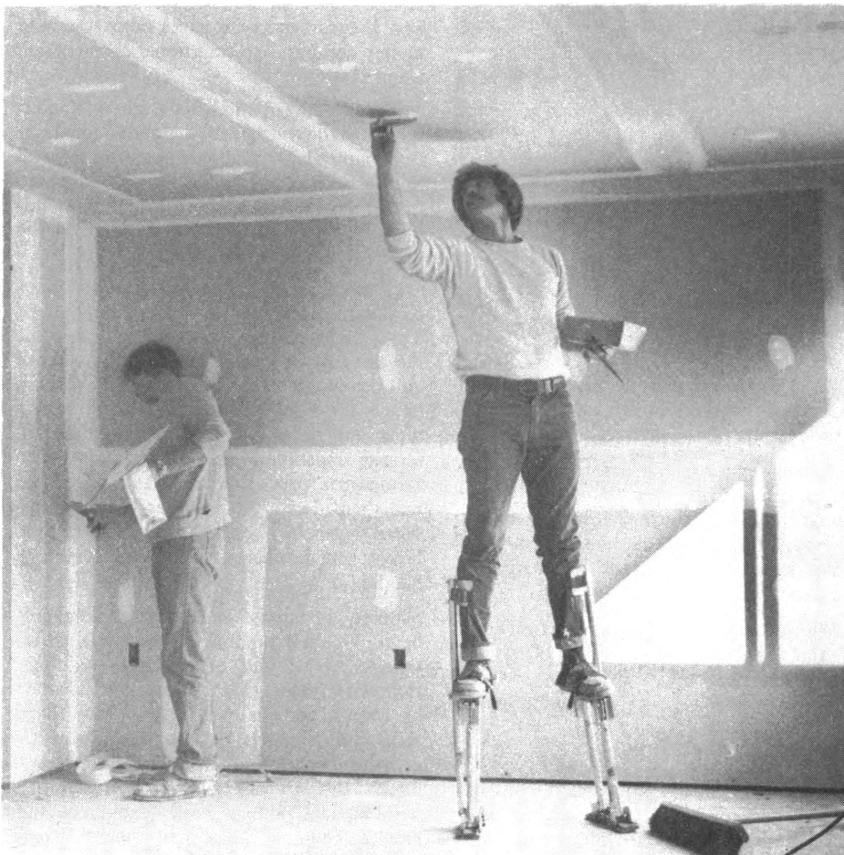
Specialty designed stilts give this finisher the added height needed to reach the ceiling.
