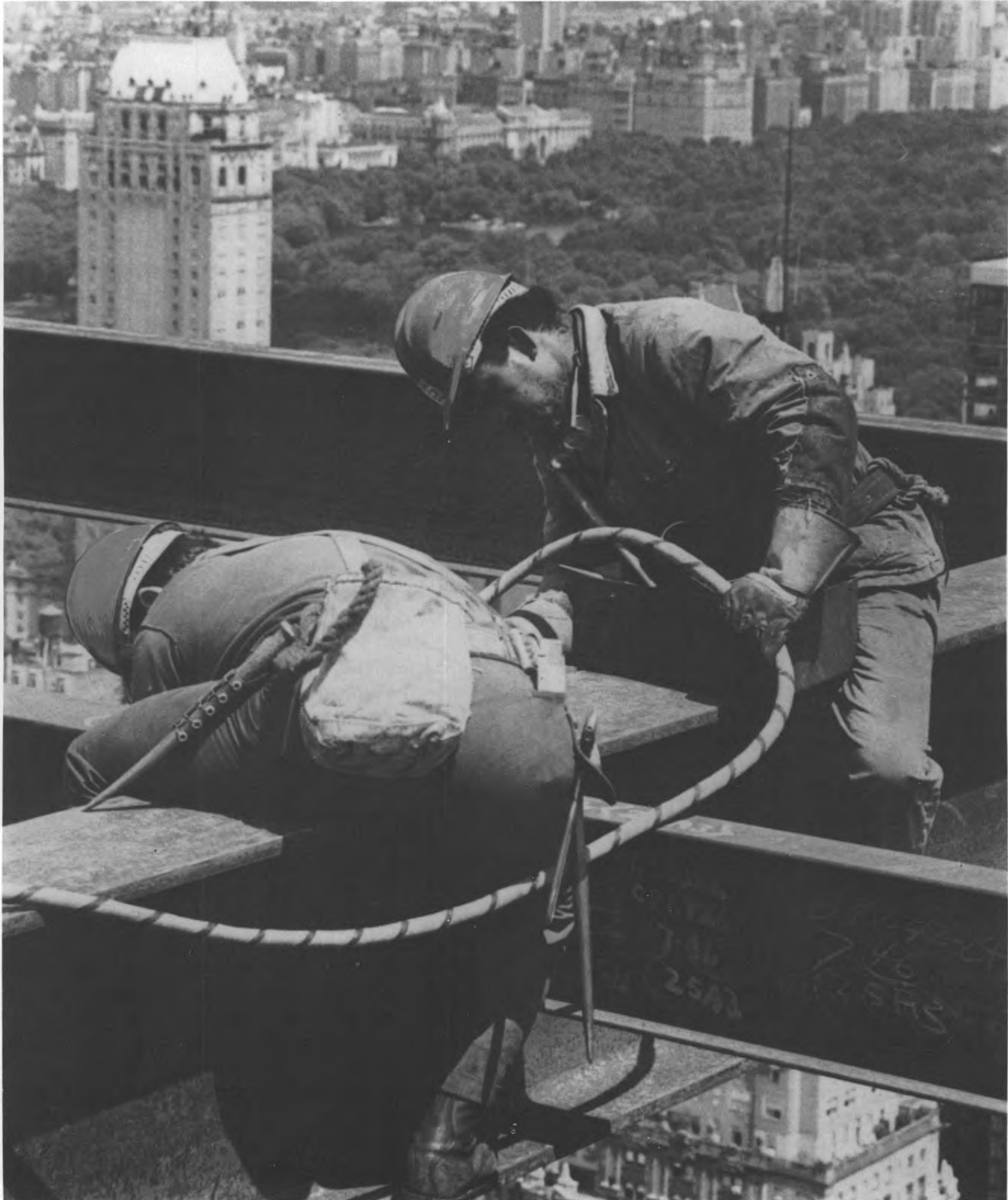
Ironworkers high above the city are protected by a system of belts and ties.
