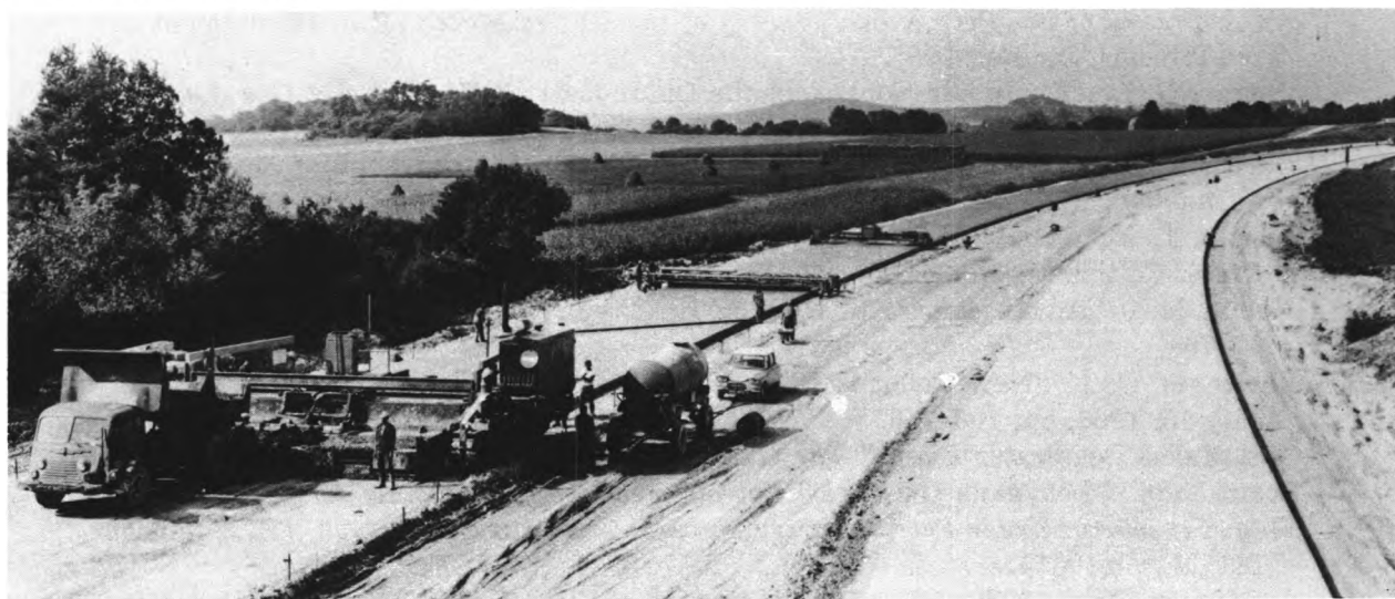
Slip-form paving machine places a continuous concrete slab for a highway without use of side forms.
