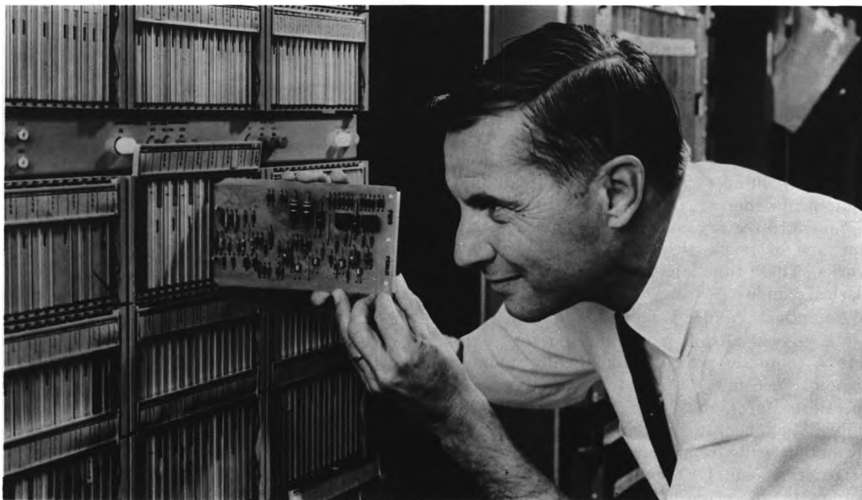
Defective circuit card is replaced in telephone electronics central office after being located by computer.
