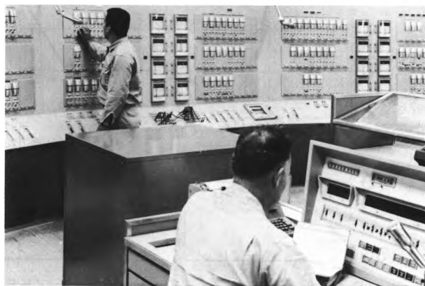
Operators oversee computer console which monitors chemical plant conditions and types out operating log sheets.
