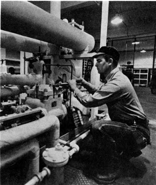
Stationary engineer adjusts a pump head.
