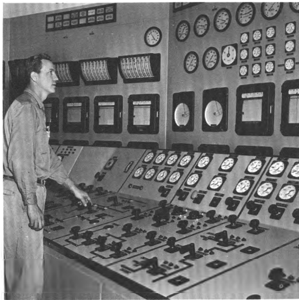
Control room operator regulates output of generating unit
