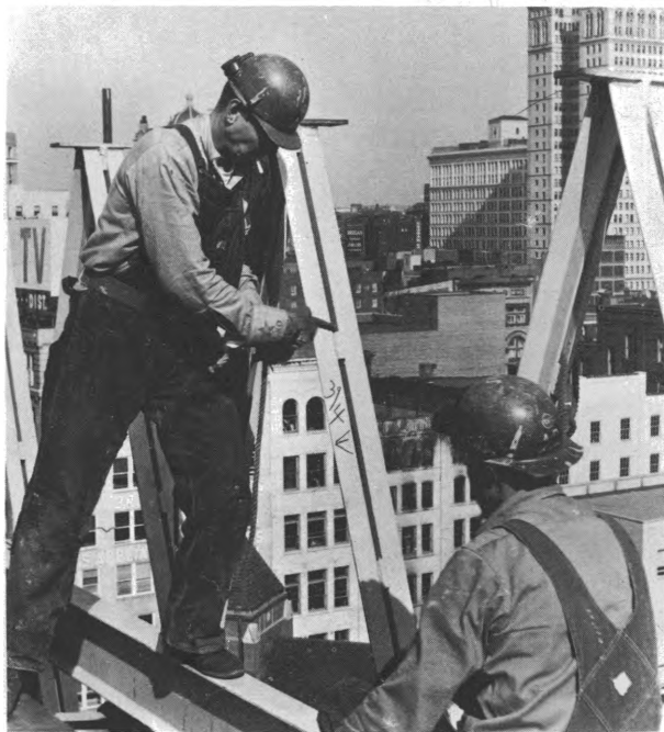
Structural-iron workers prepare for steel erection by tying safety line to framework
