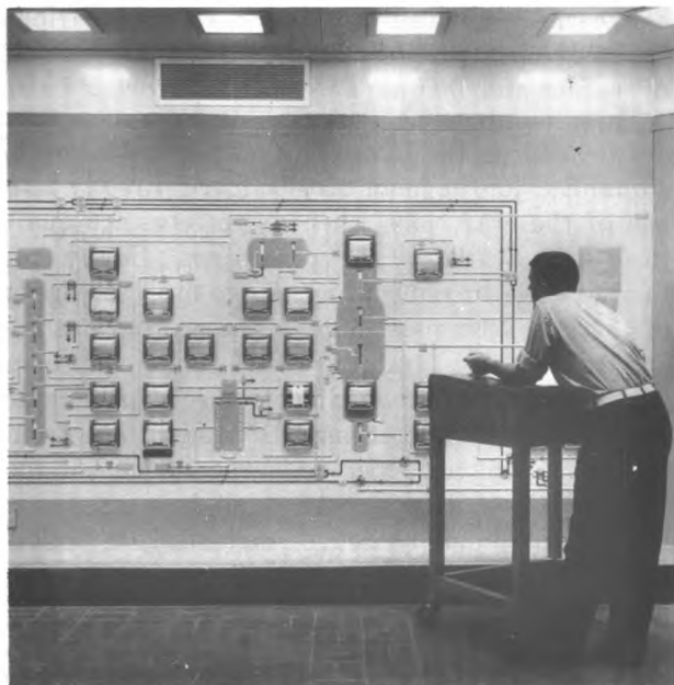
Stillman reading instruments on graphic panel which shows flow plan of entire refinery.
