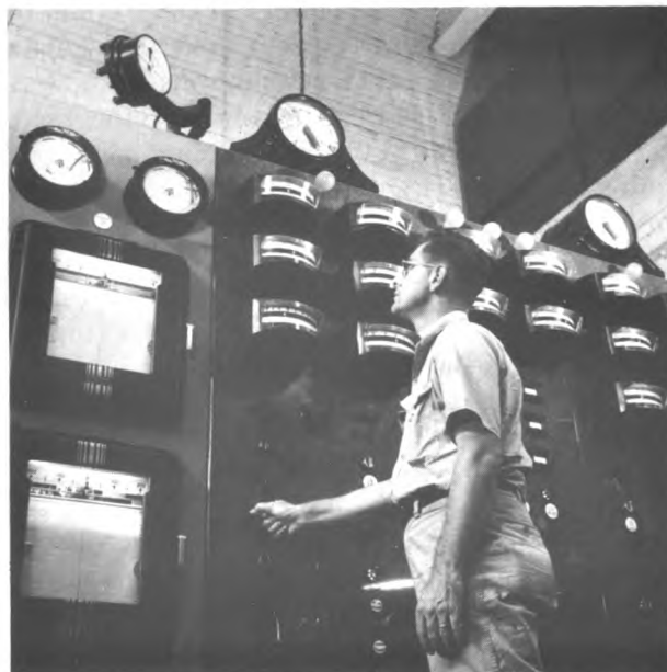
Boiler operator regulates the fuel, air, and water used in boilers by means of valves, meters, and other instruments.
