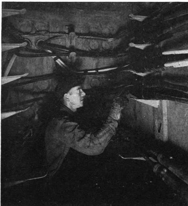
Cable splicers do most of their work in vaults beneath city streets.
