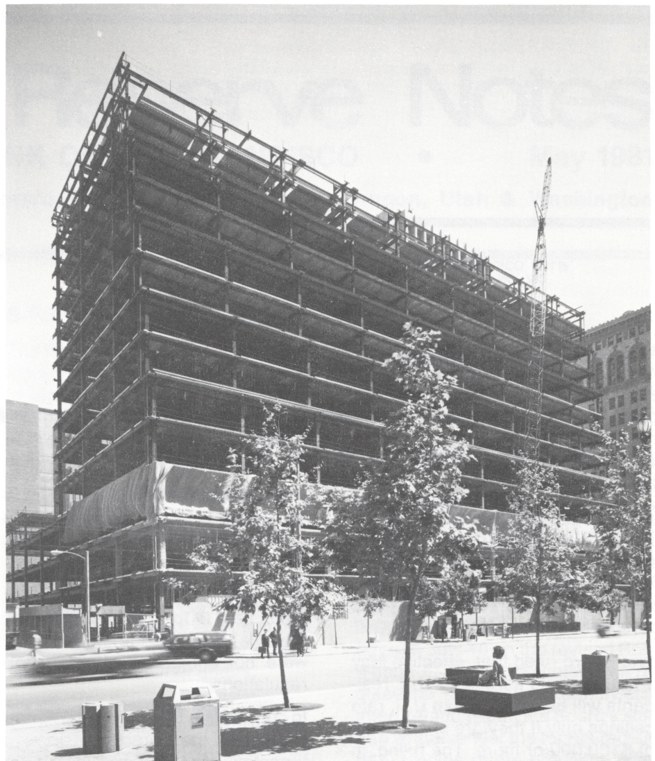
Steel work on the new 12-story headquarters building of the Federal Reserve Bank of San Francisco was completed in mid-May. The $84-million structure is expected to be ready for occupancy in the final quarter of 1982.
