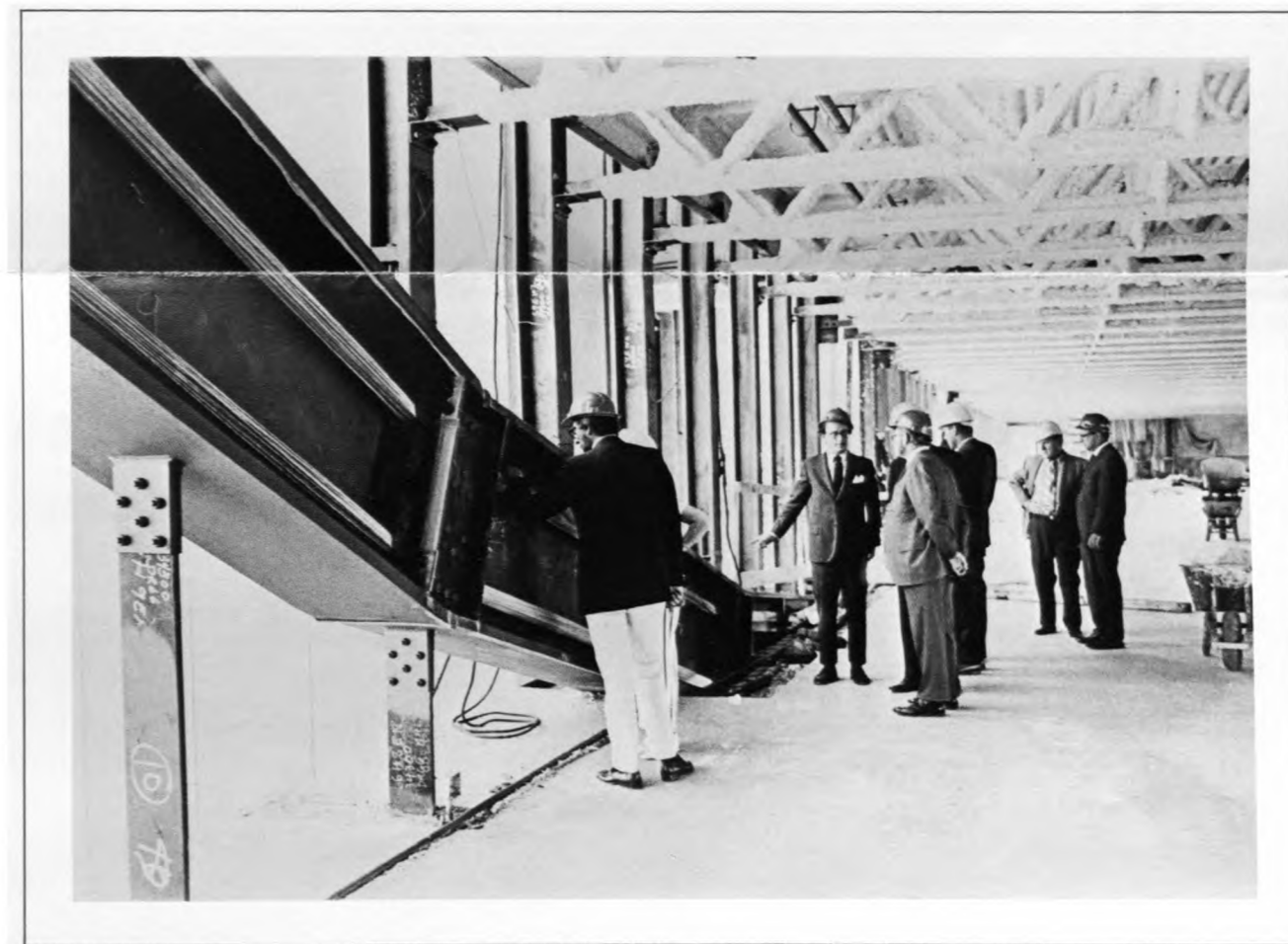
The cables and steel beam of the catenary attracted the attention of a group touring the building site last fall. Included in the group were: President and Mrs. MacLaury, John MacDonald and Roy Hughes from the Bank; architect Gunnar Birkerts and several members of his staff; and two representatives from Knutson Construction Company.
