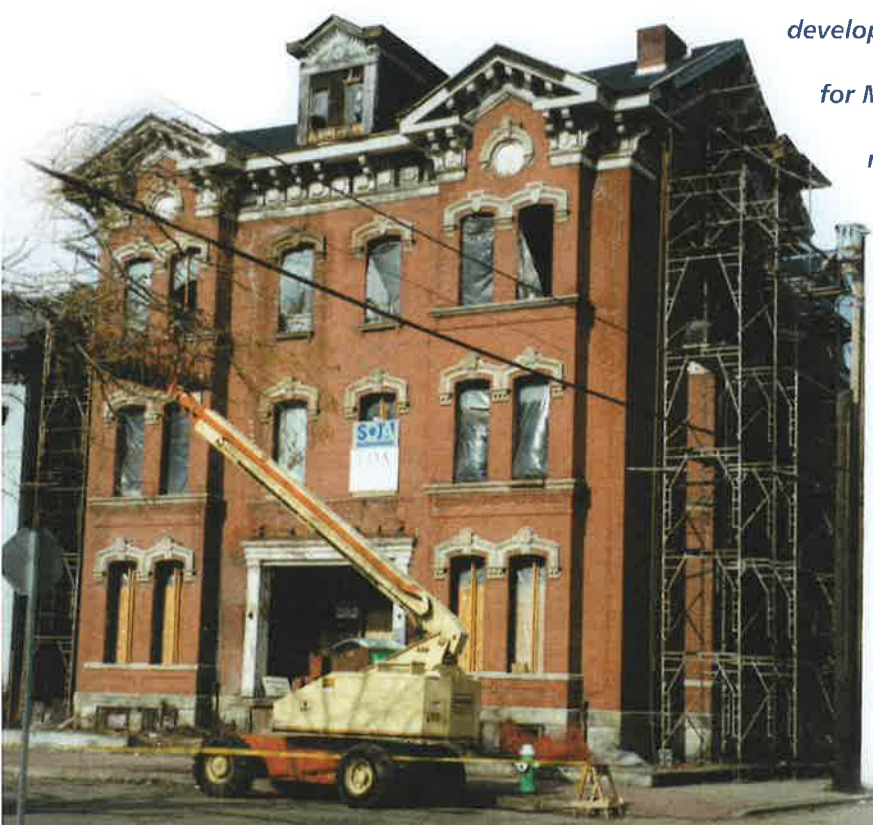
After rehabilitation, the historic Chatham Building will contain 15 units for senior citizens.
