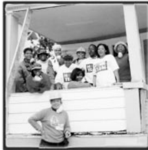
Proving that learning can take place outside of the classroom, these Mortgage Finance students help demolish a house as part of the Fannie Mae Foundation Home Team Initiative.
