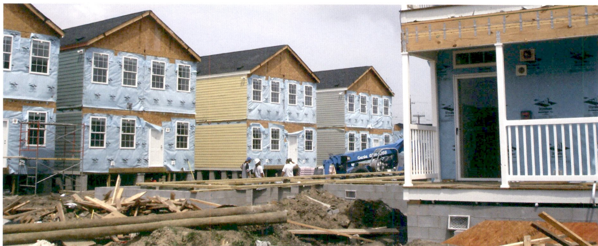
The photo shows the different phases of the Louisiana Freedmen Homes and how the development comes together quickly – from building the foundations to placing the modules and constructing the front porches after the units are in place.
