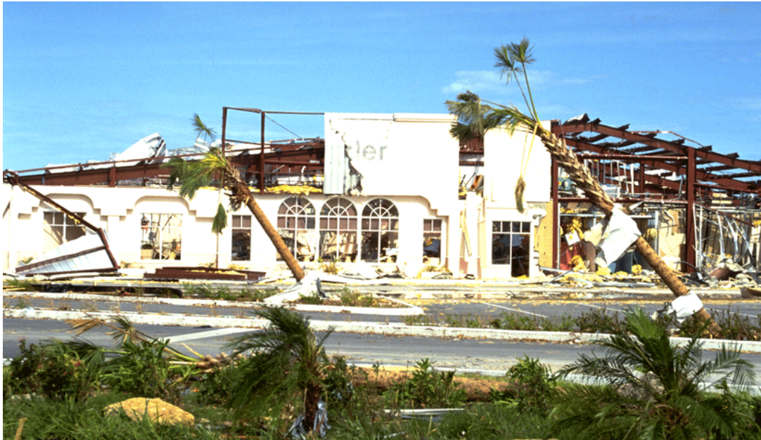
Commercial real estate in Dade County, Florida, also experienced Hurricane Andrew's fury. Photo by Bob Epstein and courtesy of the Federal Emergency Management Agency
