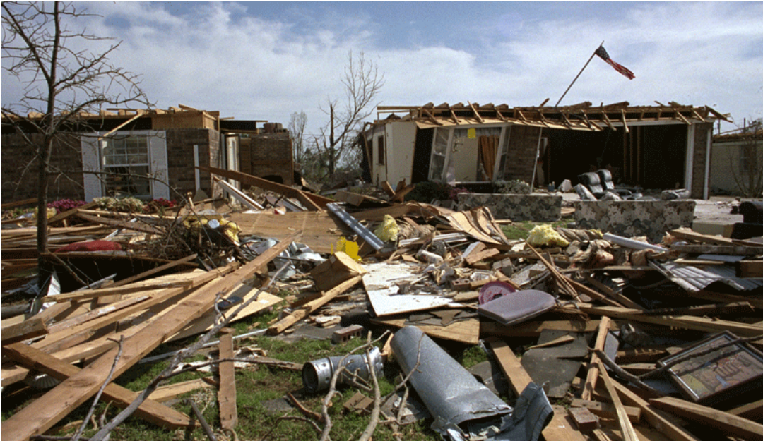
Thousands of people in South Florida suffered catastrophic loss as a result of Hurricane Andrew, as this August 24, 1992, photo shows. Photo by Bob Epstein and courtesy of the Federal Emergency Management Agency
