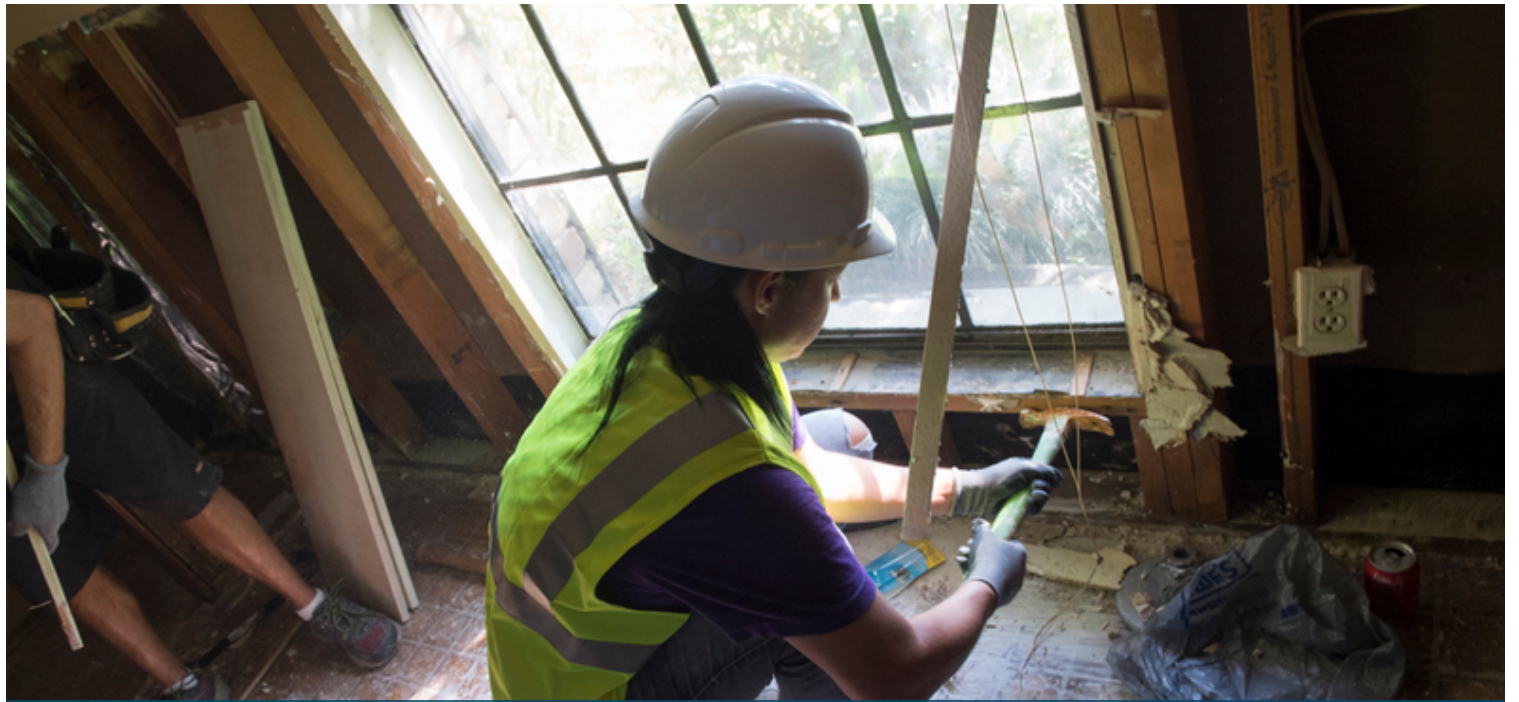
Contracted employee for the state's Shelter at Home program for flood survivors removing flood damaged debris from inside of a home in East Baton Rouge Parish. (Photo by J.T. Blatty/FEMA)
