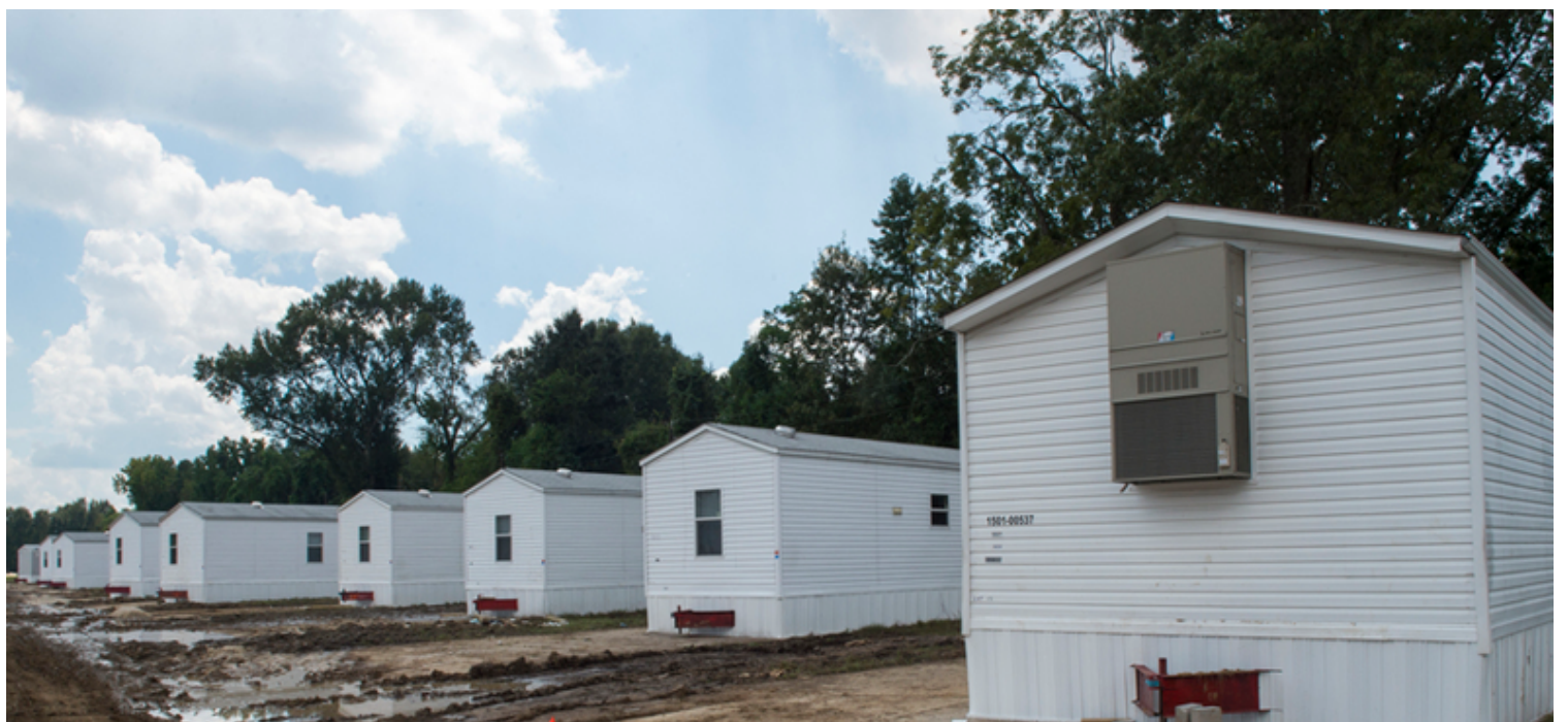
Installation of 22 FEMA Manufactured Housing Units at Leo Park in Baton Rouge for the Individual Assistance Program in response to the 2016 severe flooding in Louisiana. (Photo by J.T. Blatty/FEMA)
