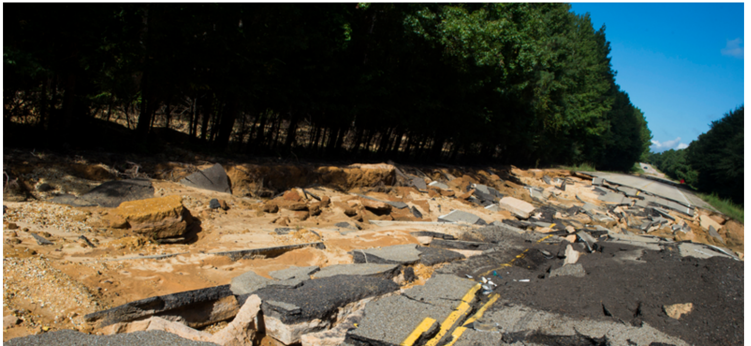
A crumbled section of LA-10 near Clinton, La, in St. Helena Parish, one month after the 2016 historic flooding. (Photo by J.T. Blatty/FEMA)
