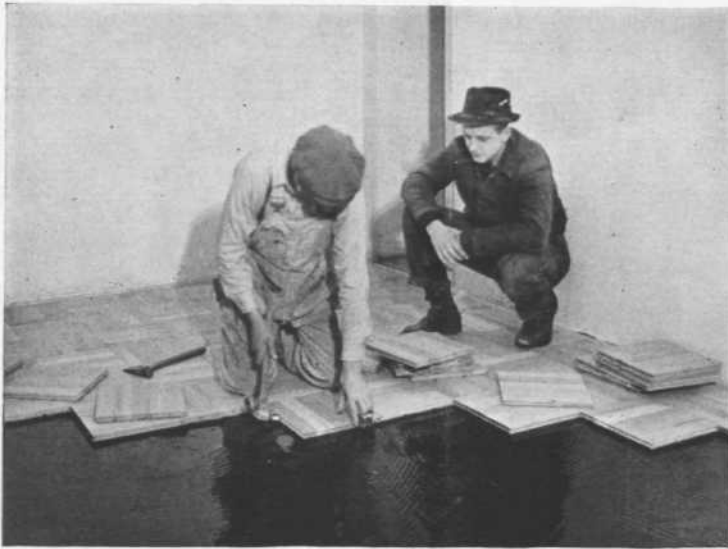
Asphalt tile has durability; in addition it comes in various shades, and there's a swing toward more color in house interiors. The floor here is being laid with tiles by Flintkote.
