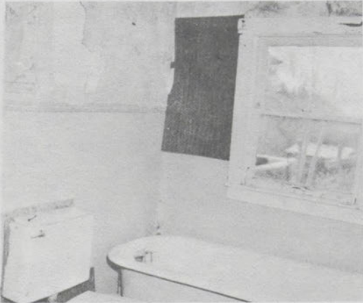
Health and safety hazard
